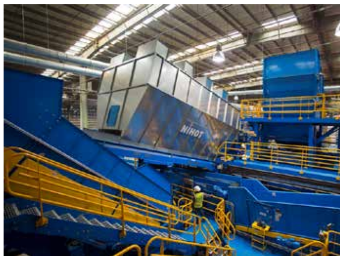
Figure 2: Bee'ah's retrofitted Material Recovery Facility
